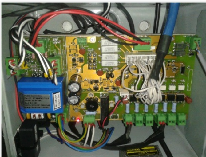
Power supply board ГНК Pump Control
